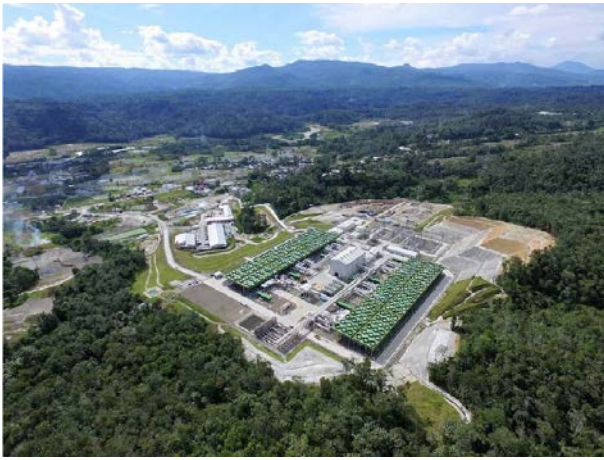
Figure 6: An aerial image of the 330 MW Sarulla geothermal power plant located in North Sumatra, Indonesia. Source: Richter (2018).
