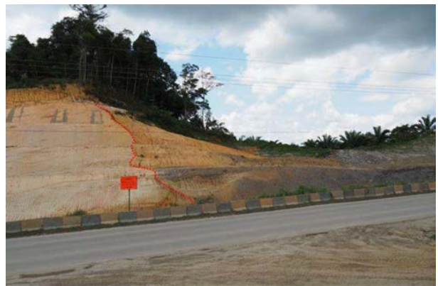
Figure 5b: Close-up of Figure 5a showing faulting (dashed red line to the right of warning panel).
