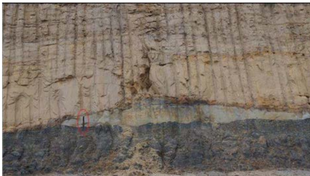
Figure 4d: Detail of erosion (with a 40 cm long knife enclosed in red circle for scale).
