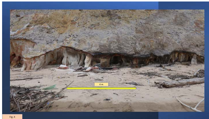
Figure 4: Scoured cliff front of the Tusan Cliff area. The ever deeper grinding sea washes out wave-cut notches. These will destabilize the cliff front until it collapses, layer by layer.
