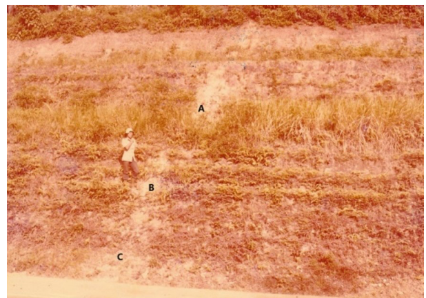
Figure 3: View of slope cut with sampling locations.
