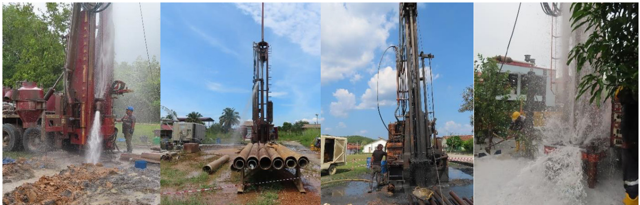
Figure 12: The figures depict drilling activities at site TW02 in Kuala Nerang, TW07 in Kulim, TW05 in Sungai Petani, and TW10 in Pendang.
