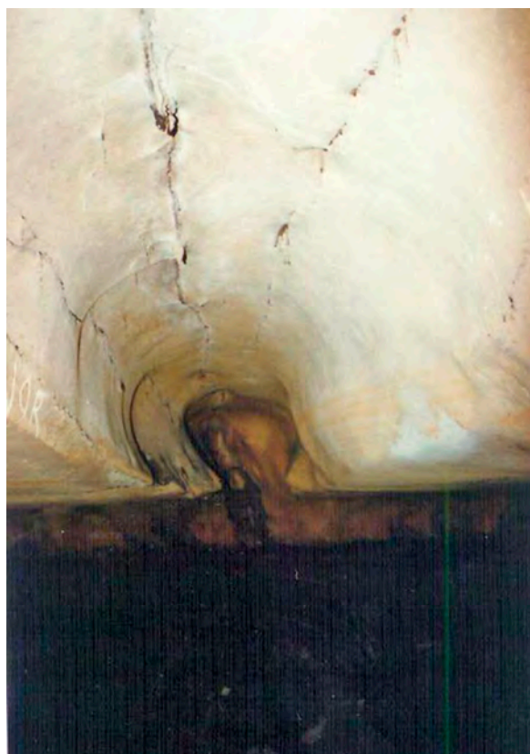
Figures 4: Bell holes found on the ceiling in Lee Ming Chamber, believed to be formed by condensation corrosion.
