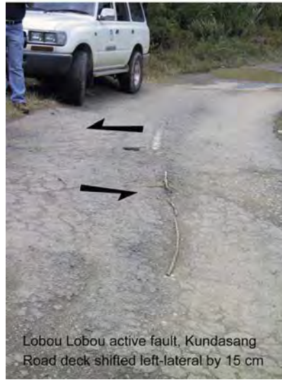
Figure 7: Active strike-slip faulting on the Lobou-Lobou segment of the Crocker fault zone in the vicinity of Kundasang; photograph taken on 19 July 2006.
