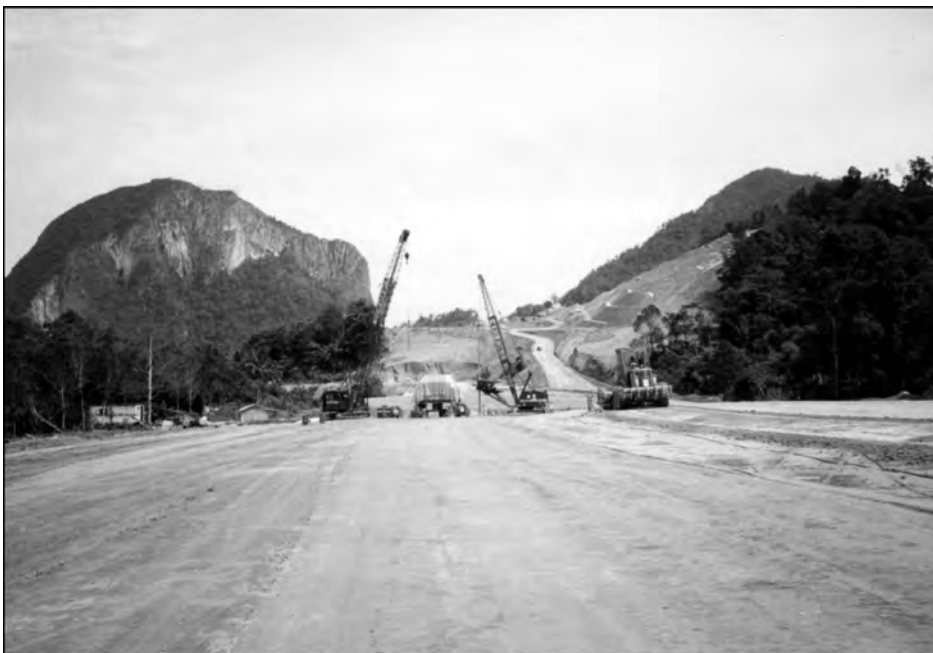
Figure1: North-South Highway under construction, looking north. G. Tempurung (limestone) on the left, schist in cut-slope on the right, and granite further right (Main Range). Colluvium occurs along the Highway mainly as valley fills.
