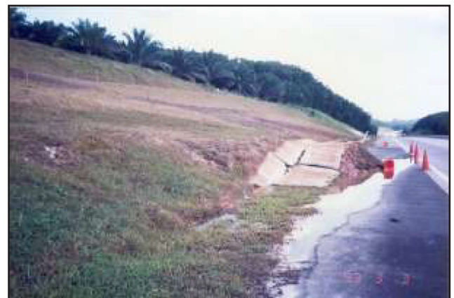
Figure 14: “Flattened” cut slope in graphitic schist, N-S Highway near Rawang.
