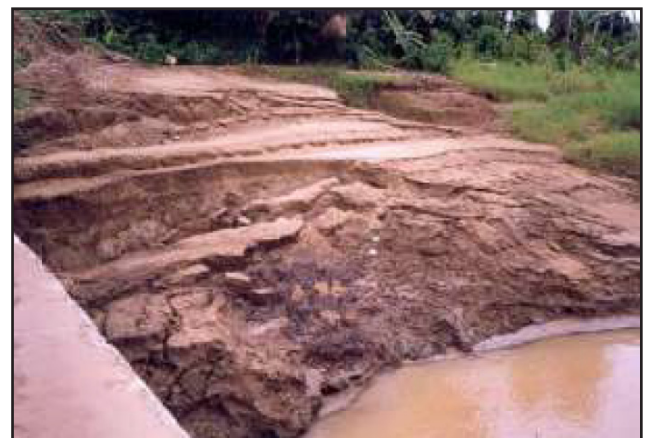
Figure 23: Riverbank instability, Sarawak.
