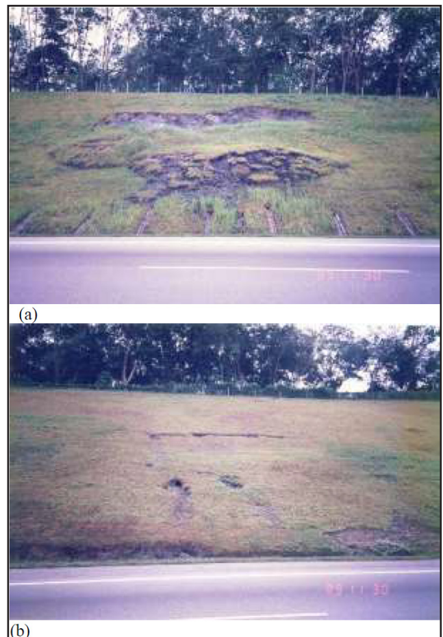
Figure 12a, 12b: Graphitic schist soil slope failures, Senawang-Ayer Keroh Highway.
