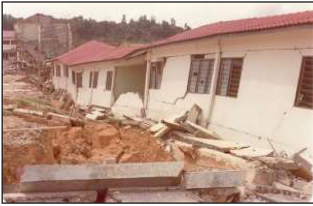
Figure 24: Rapid draw-down of mining pond triggering slope failure and destroying houses, Kuala Lumpur.
