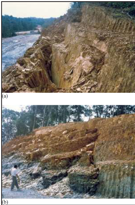
Figure 15a, 15b: Slope failures controlled by bedding planes and faults, Sarawak rural road.
