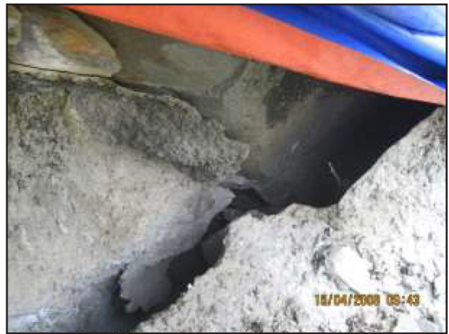
Figure 19a: Opening of sub-vertical joints in sandstone due to toppling failure, Bakun Dam, Sarawak.
