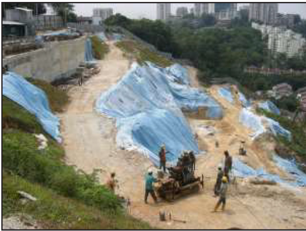
Figure 26: Housing development on slope underlain by the Kenny Hill Formation, comprising interbedded quartzite and phyllite, Kuala Lumpur.
