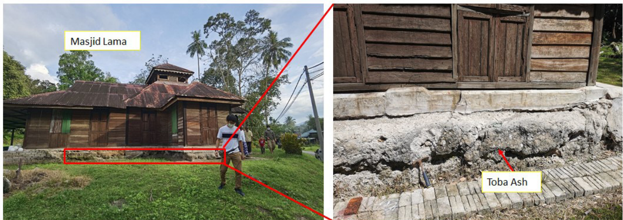
Figure 4: Exposed Toba ash as basement of Masjid Lama at Kampung Chepor, Lengong.
