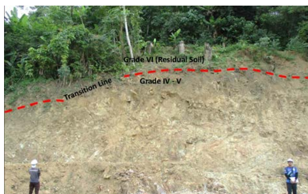
Figure 8: Overview of weathering profile of grade IV – V at circle C area of Figure 2.
