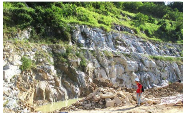
Figure 4: Overview of weathering profile of grade II – III at circle A area of Figure 2.
