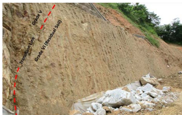
Figure 10: Overview of weathering profile of grade VI (residual soil) at circle A area of Figure 2.
